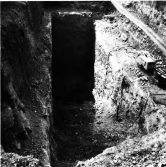
Photo. 3. The Pump house
